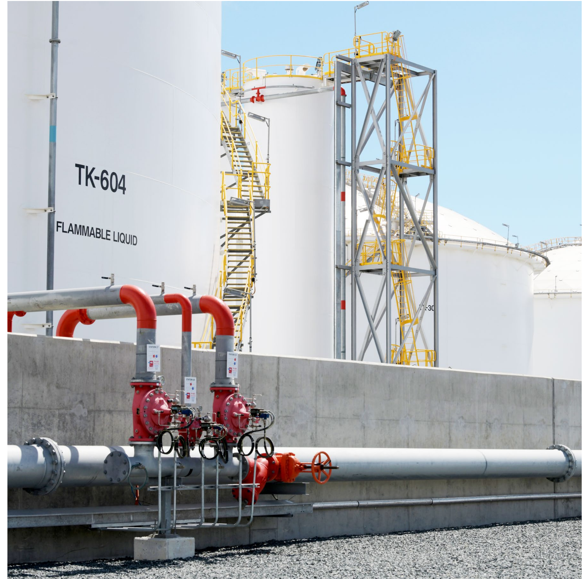
Impala Terminals, Kwinana, Australia
